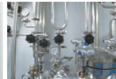
CIP&SIP Ensure the sterility of the whole manufacturing process
